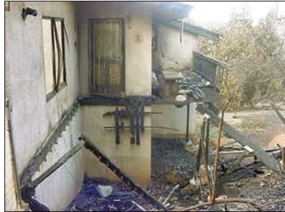
Figure 5. Combustible debris under this deck ignited and led to the destruction of the deck. Although the siding is noncombustible, the fire spread from the deck through a window to the interior (firecenter.berkeley.edu).
